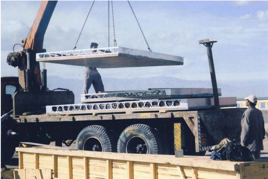
ThermAlloy Composite (Steel & Concrete) Precast Panels are unloaded at the project site by Mammut Building Systems.
