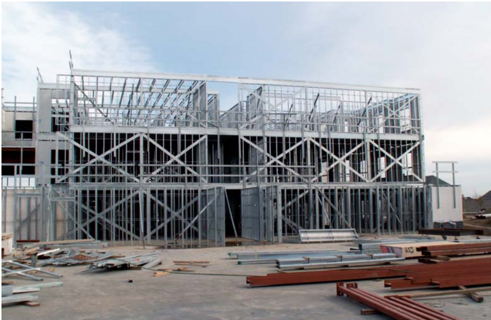
This 3-story commercial structure in Edmonton is framed in light gauge steel products manufactured by Steelform Building Products Inc.
